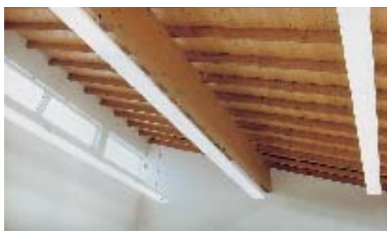
Daylight-dependent control of the rows of luminaires in the workshop
