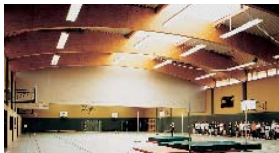
Apart from the lighting, further functions in the gym such as opening/closing the dividing curtain and lowering the ropes are controlled via the EIB
