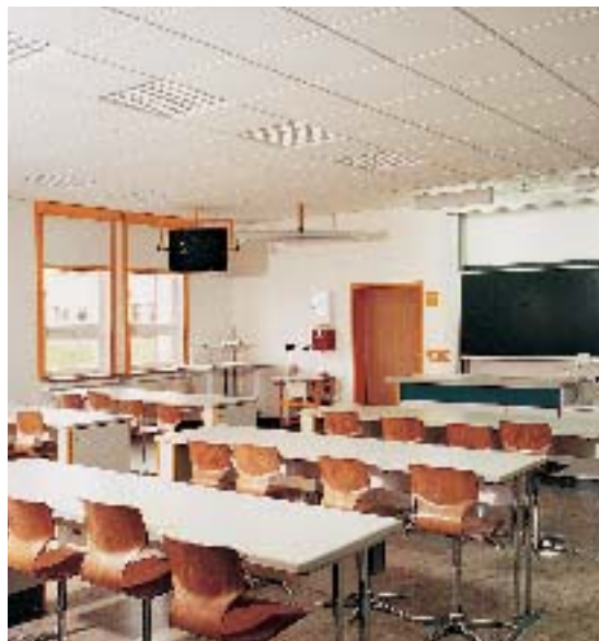
The lighting control in the classrooms can be carried out centrally and manually on-site. The lighting is also operated as brightness- and time-dependent
